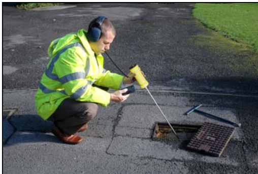
Leak Sizer use for direct leak listening
